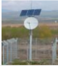
VSAT (satellite communication)
